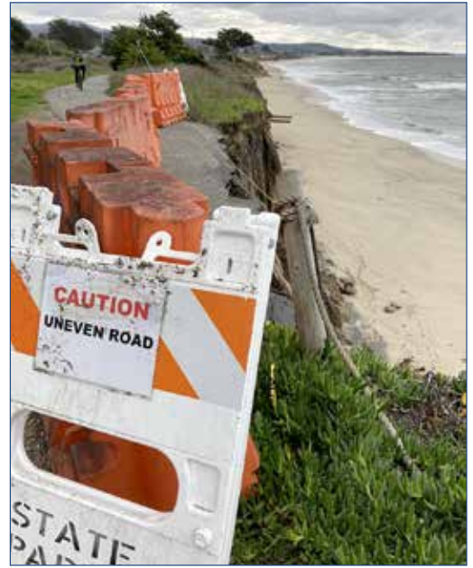
Collapsed trail south of Miramar
