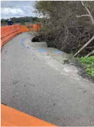
The road was undercut by a creek that flows there causing most of the road to collapse.
