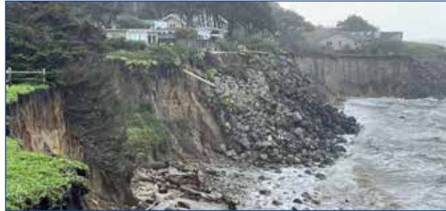
This photo shows the accelerated erosion on bluffs in Moss Beach when adjacent areas are armored with rip-rap (boulders). The bluffs in the foreground lost about 10 feet in January 2023. Photo: Steven King
